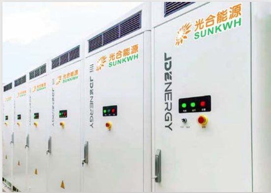
📍 Mocai Energy Storage Project 🔋 ESC:1039.6kW/1145kWh
